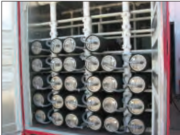
FIGURE 3. The air-separation modules shown here are for a nitrogen-production unit
